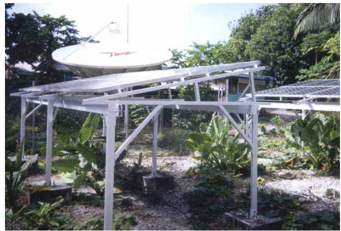
Figure 4-2 – USP Solar Installation Atafu
